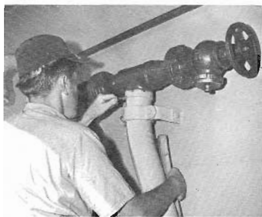
"If I can just keep this hole plugged until they secure the water"
